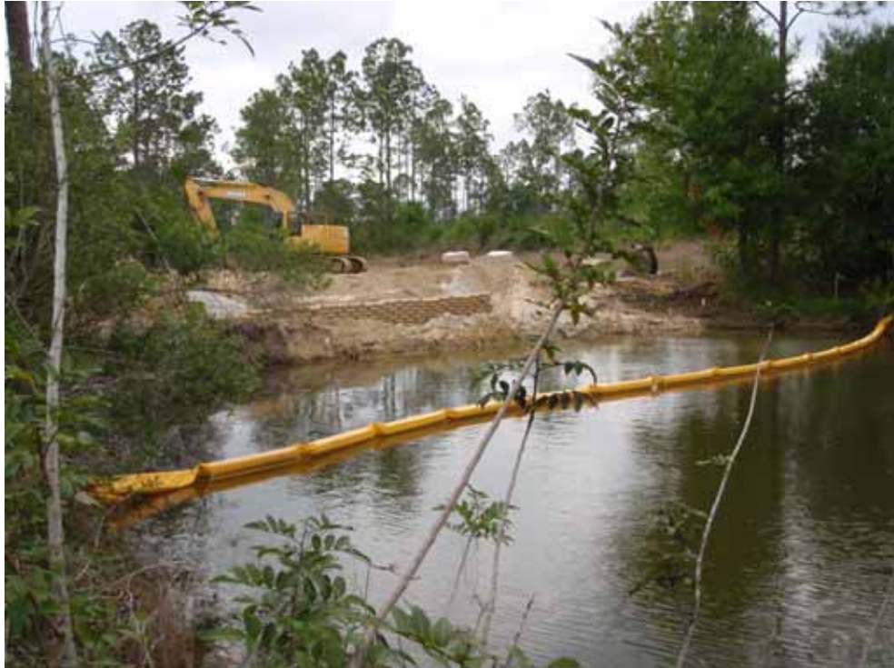
Photo #4. The contractors have placed concrete type bags as a reinforcement wall.
