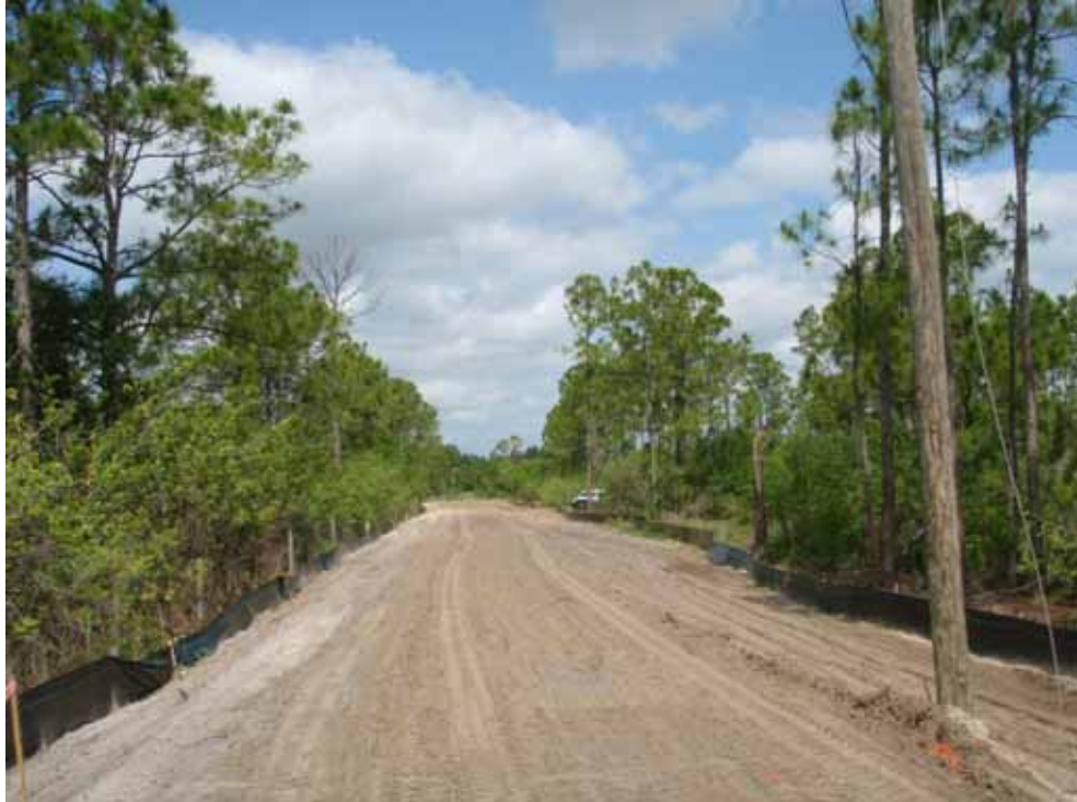
Photo #7 is the southern berm at grade, smoothed out and rocks removed.
