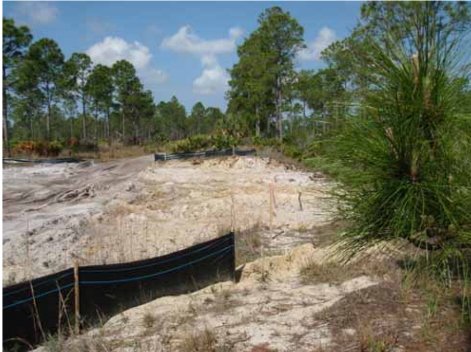
Photo #3 if you look closely on the left side, the shallow flowway has been excavated.
