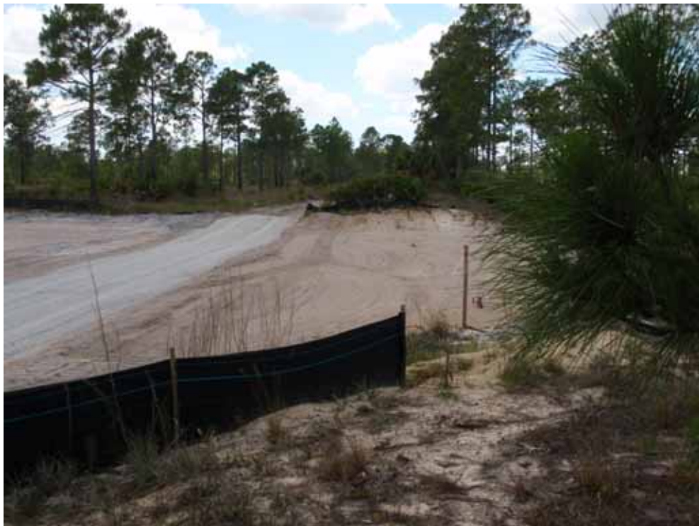
Photo #3. The flowway is complete and they have installed an equestrian crossing that will give the horses firm footing while crossing the wetland.
