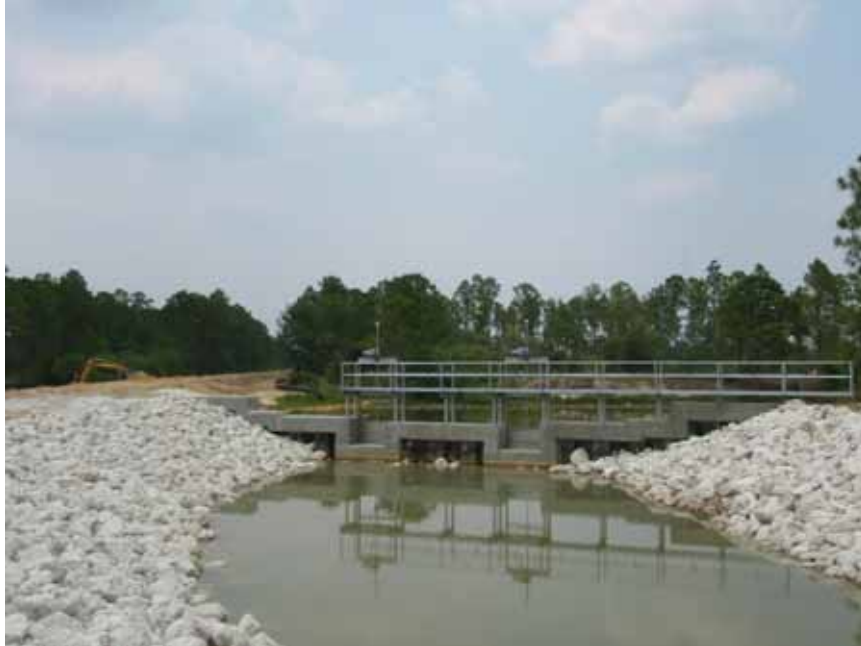
Photo #6 the weir is complete and tons of rip-rap (rocks) have been installed on the banks to stabilize the soil. The rocks also work to slow down the water flow so that the water doesn't carve a hole into any of the banks.
