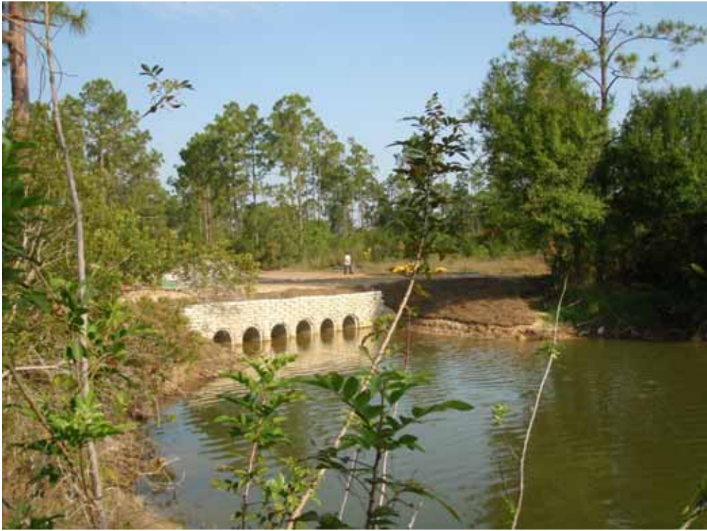
Photo #4. The connection between the "nose" of dolphin pond and the rest of the ponds is complete.
